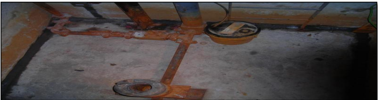
Figure 4. Ill effect of seawater intrusion on pipes laying below ground
